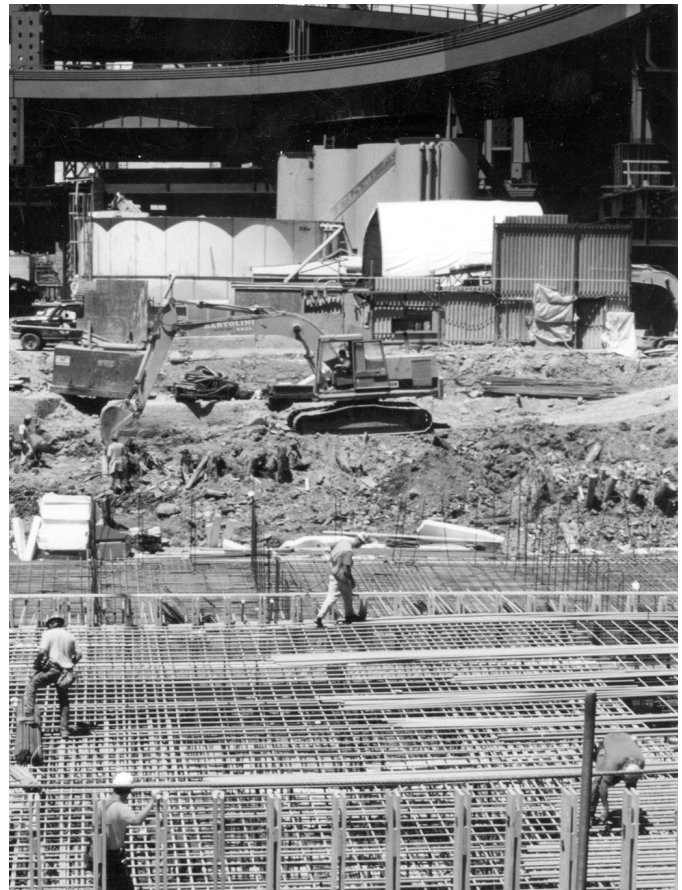
“The telltale sign of imminent pouring of concrete is the laying of green metal mesh. Here, the roadbed from the tunnel upward to the bridge is prepared to accept the concrete. This picture was taken from the sidewalk on Causeway Street. The Fleet Center is just out of sight to the left.”
