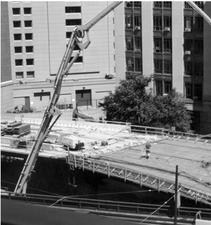
“Sometimes concrete has to take roundabout way when being poured. Here, the Leverett Connector to the Zakim Bridge is getting it’s concrete from below, pumped up through a series of plastic pipes. The Registry Building passively awaits its demise.”
