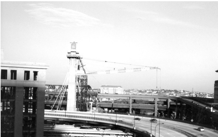
At 240 feet, the Cornell tower crane is one of the tallest free-standing tower cranes in the U.S.
